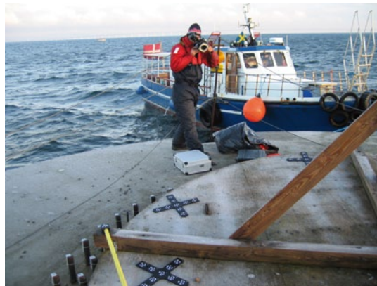
Fig. 10: Measurement and inspection of 120 mounting bolts with the TRITOP CMM system on high seas
