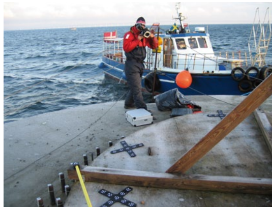
Fig. 10: Measurement and inspection of 120 mounting bolts with the TRITOP CMM system on high seas
